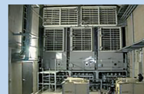
NO 2 Removal System
