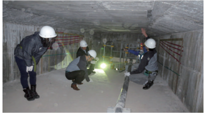
Observation of PC (pre-stressed concrete) beams, Gerber part, renovation construction March 14, 2017 Route 4 Shinjuku Line, Sendagaya overhead box girder
