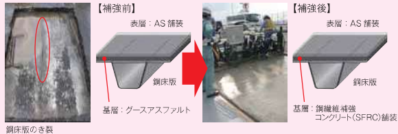
鋼床版のき裂
