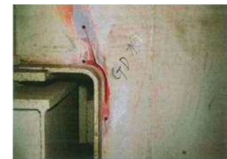
鋼桁の疲労き裂
