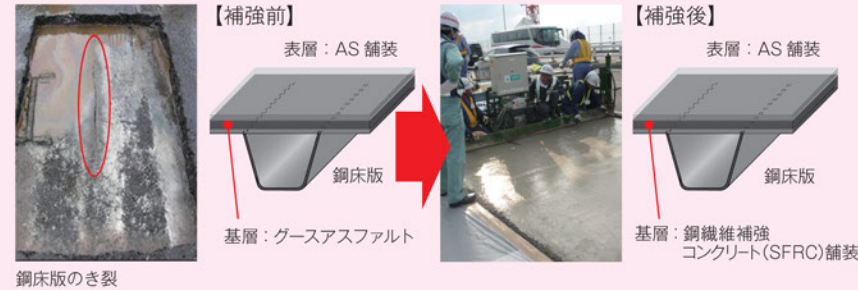
鋼床版のき裂
